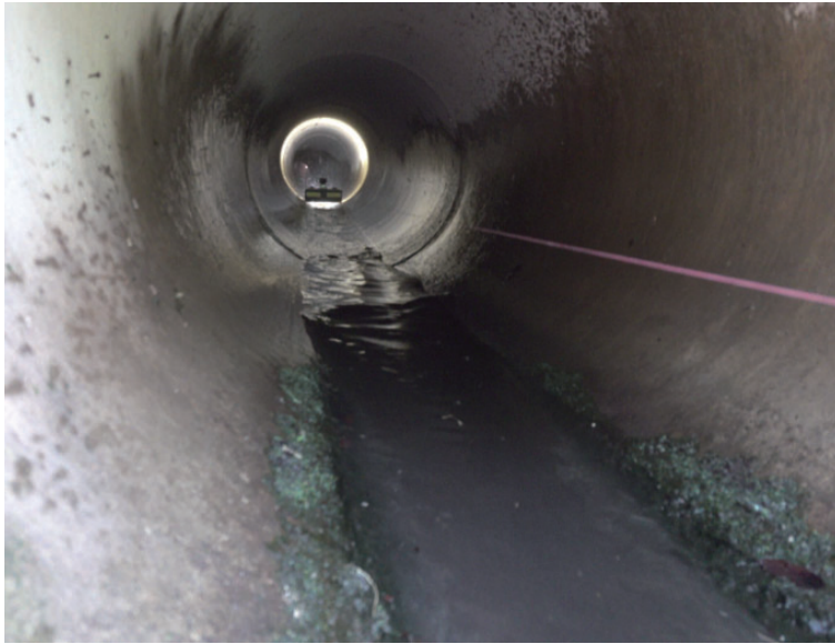
Fi4 flies through the pipe at the speed up to 3m/s, enabling fast and efficient video shooting.
